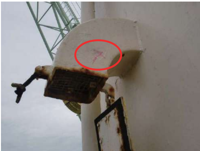
Hole with inappropriate repair with tapes
