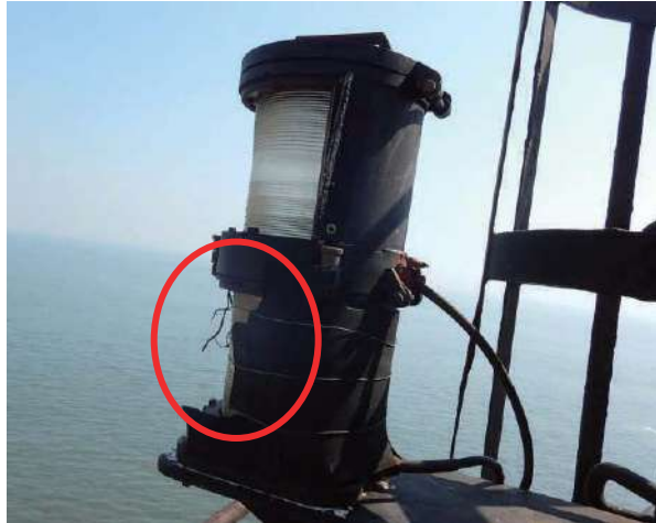
Damaged navigation light
