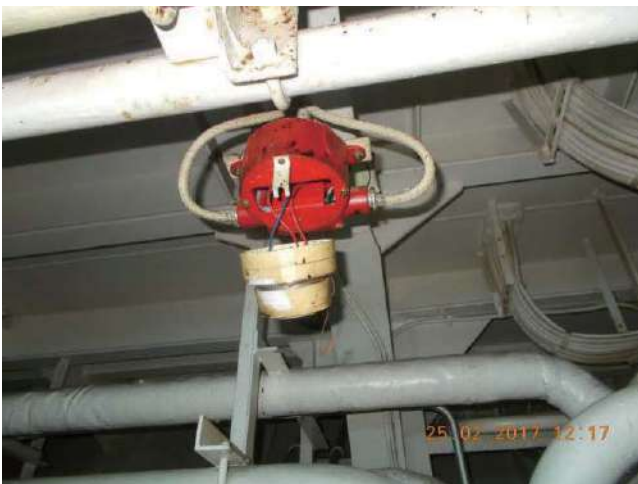
Defective of fire detector
