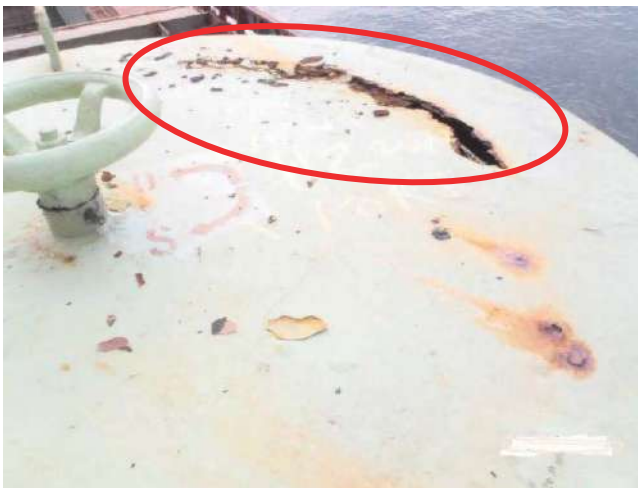
Corrosion holes in the casing of ventilator
