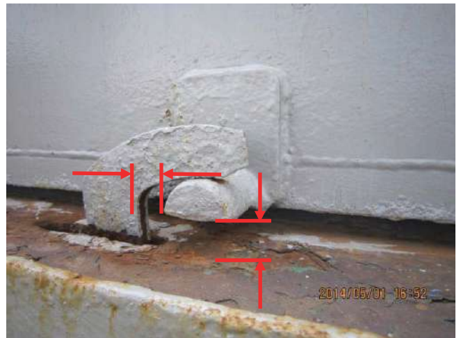
Excessive gaps of hatch cover
