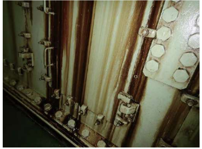
Oil leakage of M/E
