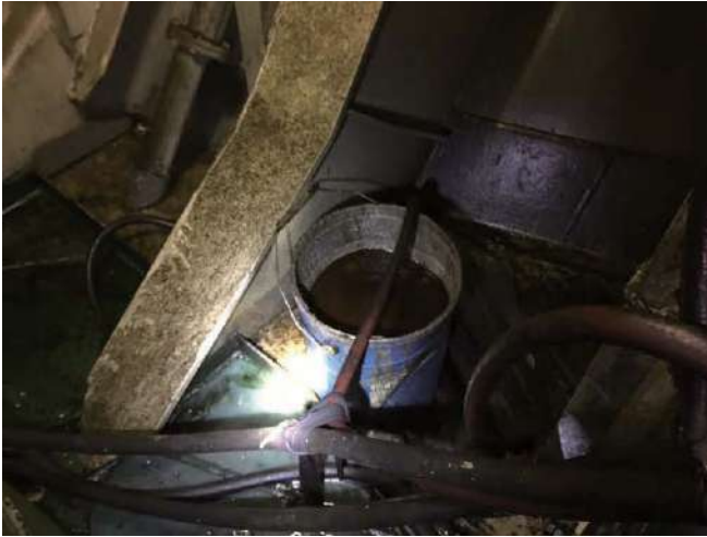
Bucket filled with oily mixture bilges in E/R
