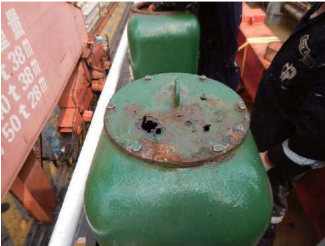
Corrosion holes in air pipe head
