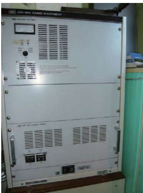
Switch Panel for MF/HF radio
