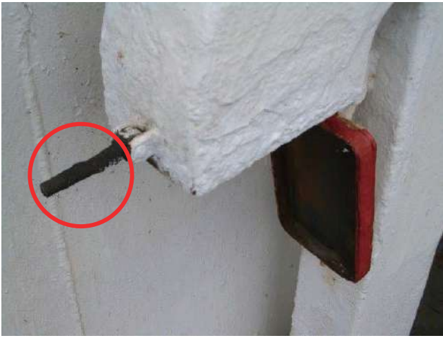
Missing butterfly nut of gooseneck ventilator
