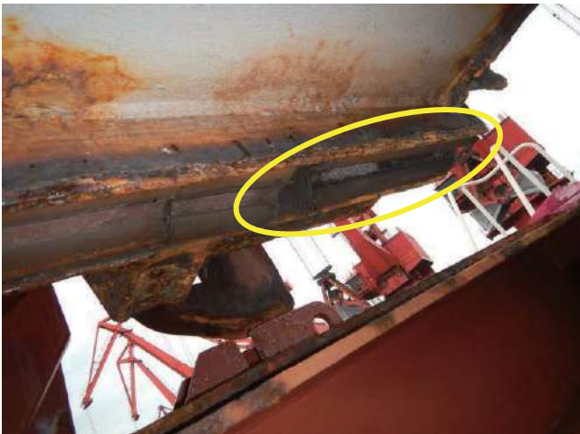
Partly missing rubber packing
