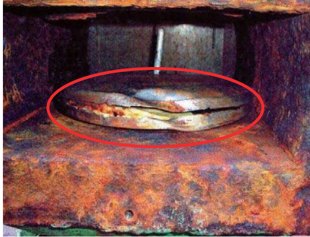
Damage of disk float
