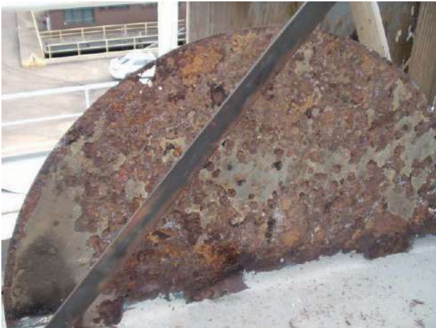
Wastage/Corrosion holes in fire damper flap
