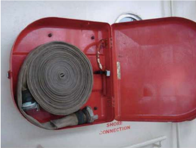
Missing of fire nozzle
