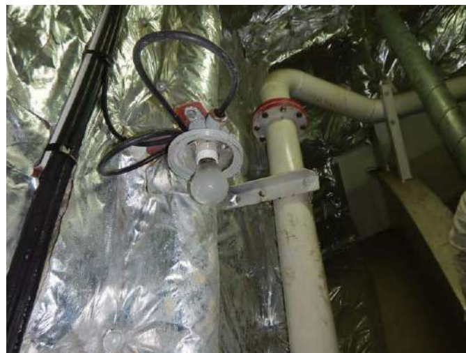
Missing of guard of lighting fittings in E/R
