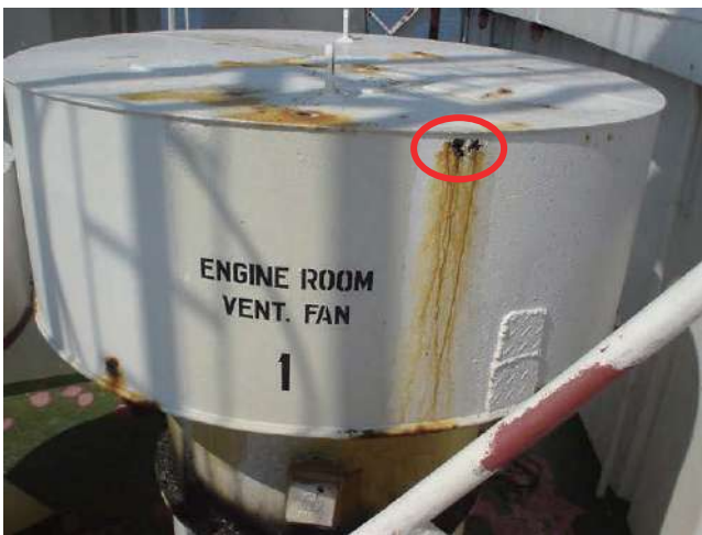
Corrosion holes in the casing of ventilator
