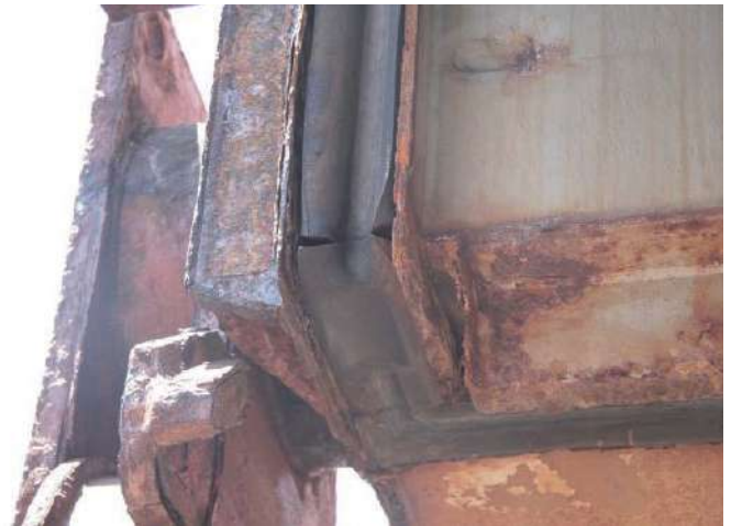
Deteriorated and cracked rubber packing
