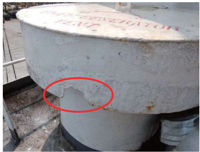
Wastage of the casing of ventilator
