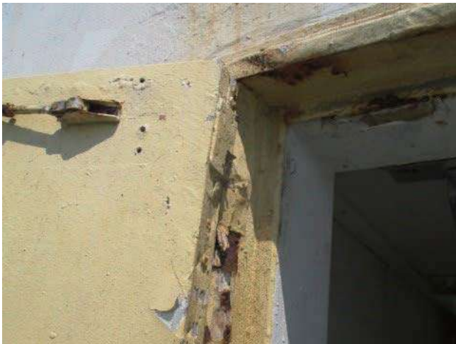
Wastage of door and door frame
