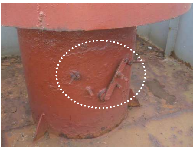
No marking of “Open-Shut”
