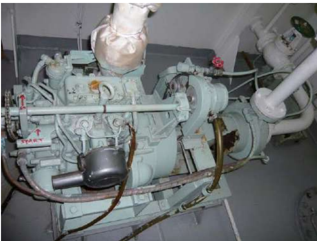
Emergency fire pump
