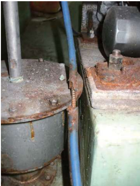
Defective release cable
