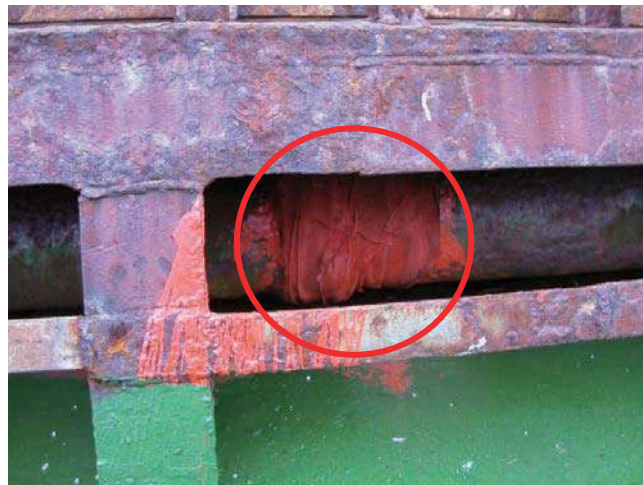
Inappropriate repair by cloth
