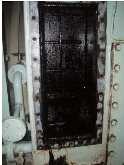
Oily inside of oil water separator
