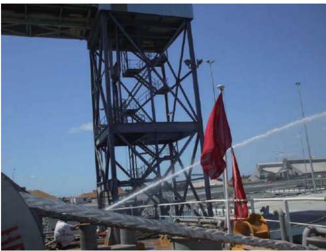
Performance test of emergency fire pump
