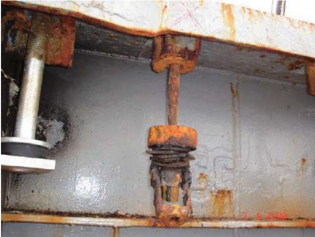
Wasted securing device
