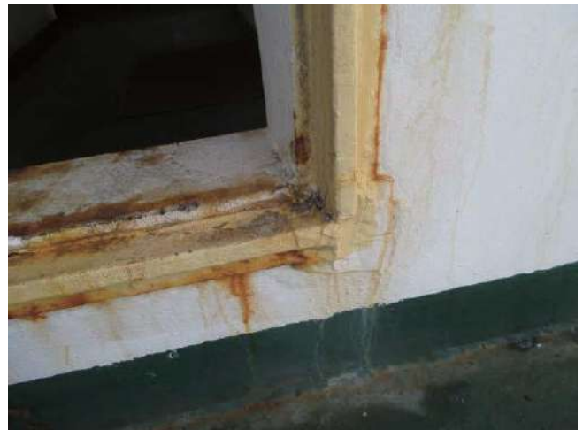
Wastage of door frame
