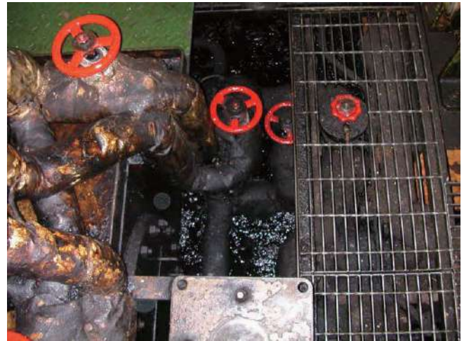
Dirty Engine room tank top
