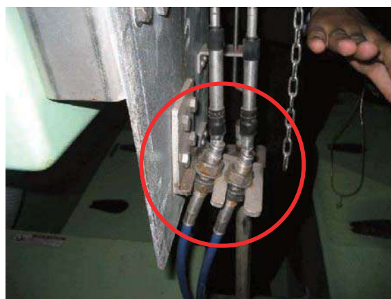
Bent release cable and bracket
