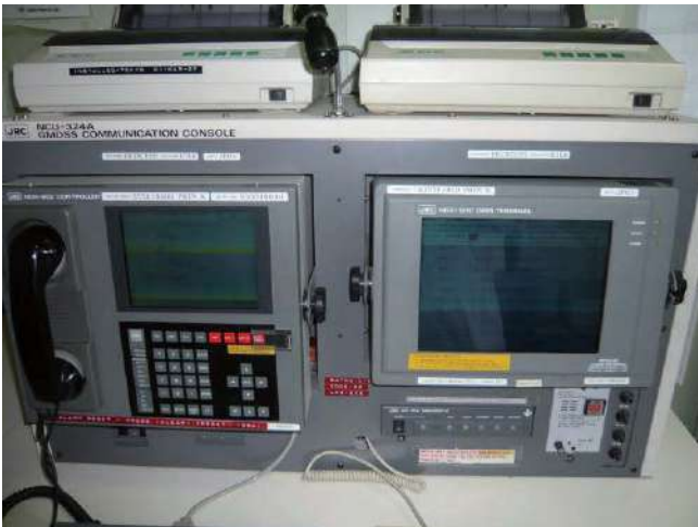
GMDSS communication console
