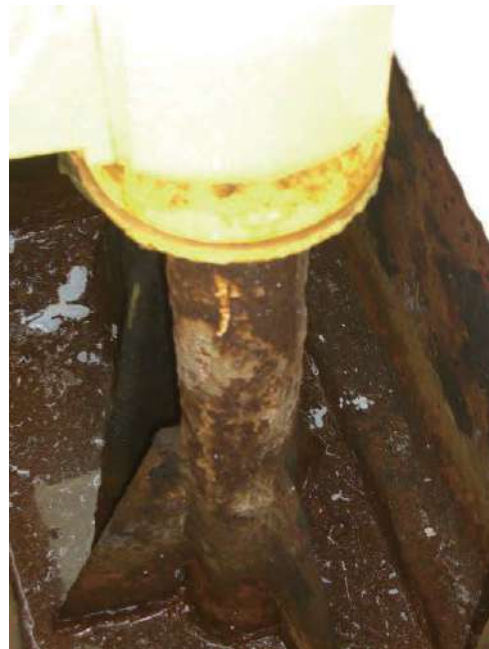
Wastage of air pipe
