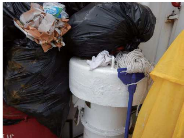
Ventilator is obstructed by garbage
