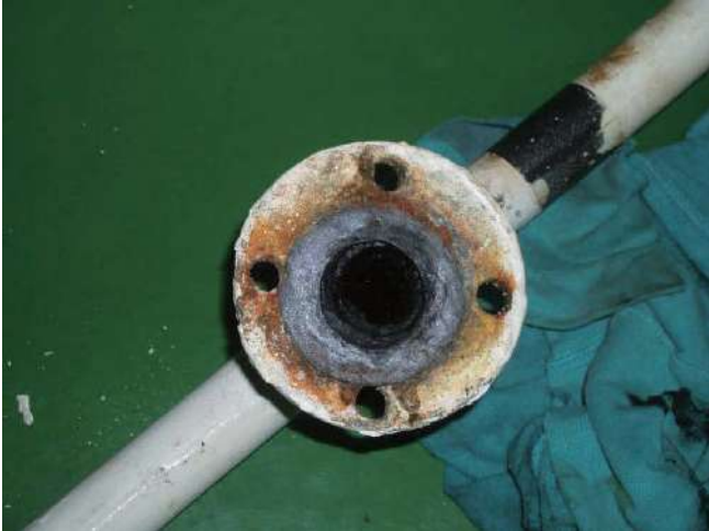
Oily inside of discharge pipe
