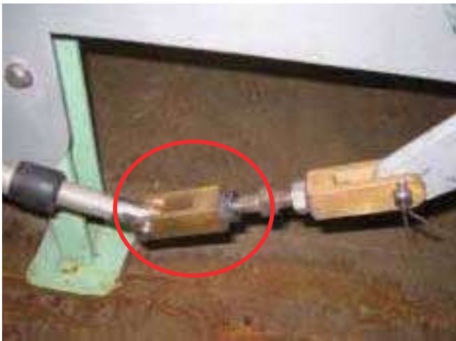
Incorrect condition of turn buckle
