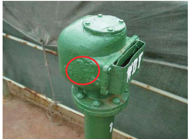
Inappropriate temporary repaired by putty
