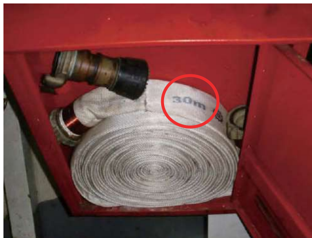
Length of fire hoses in E/R is not to be more than 15m
