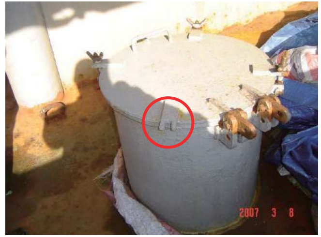
Missing nut and bracket with bolt
