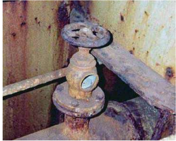
Missing of coupling
