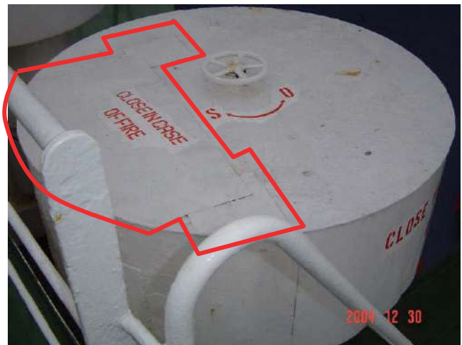
Inappropriate temporary repair by tape
