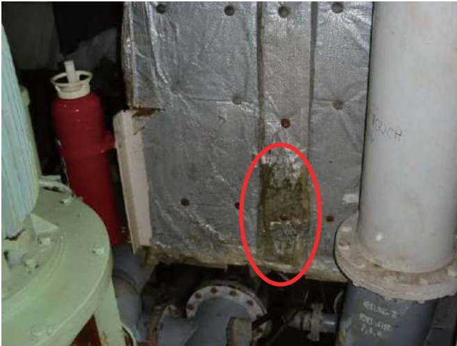
Partly missing A-60 class insulation
