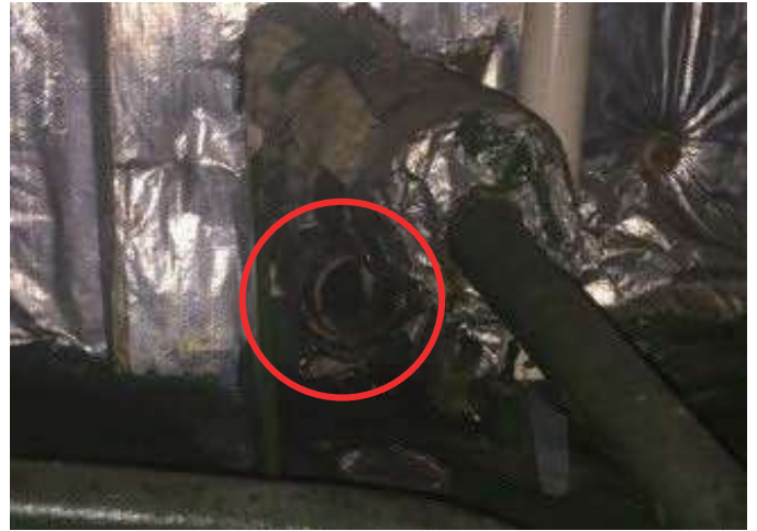
A hole on the A-60 class bulkhead
