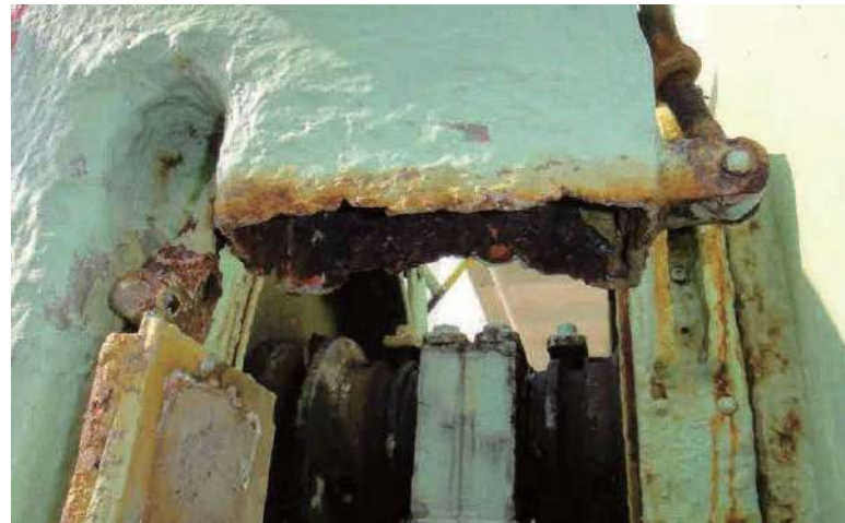
Wasted gooseneck ventilator
